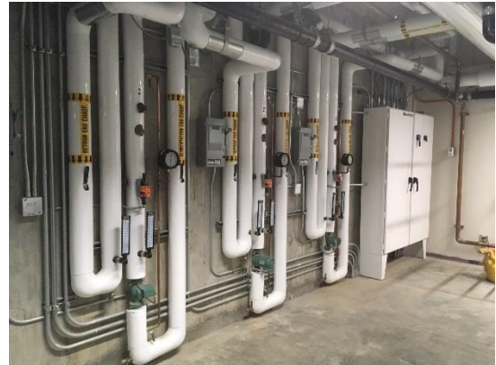
Heating mixing groups in basement
